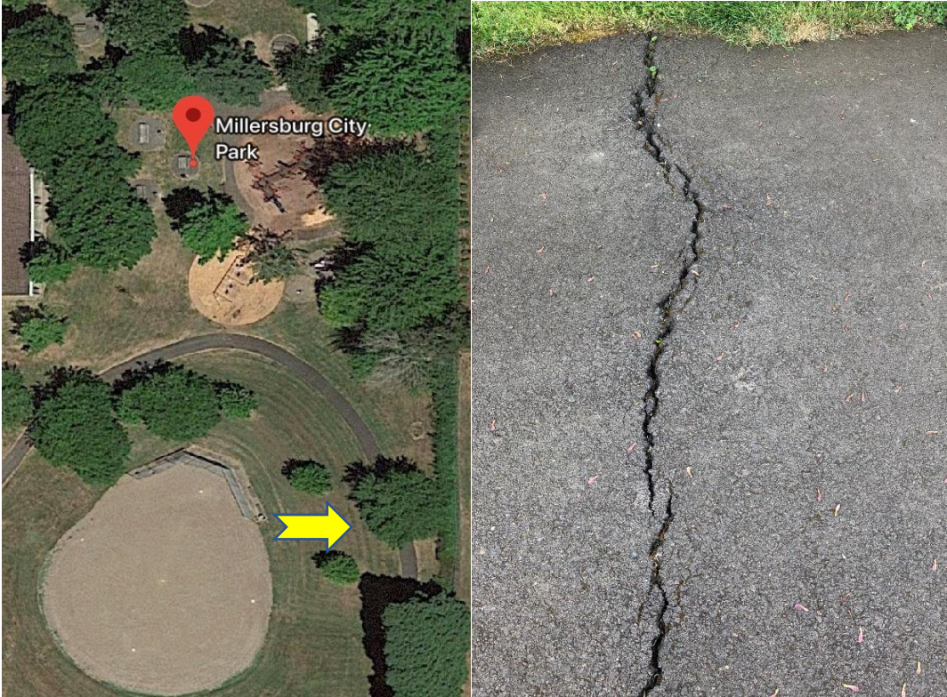
Exhibit A: Millersburg Park - Root upheaval in sidewalk, southeast of playground.
