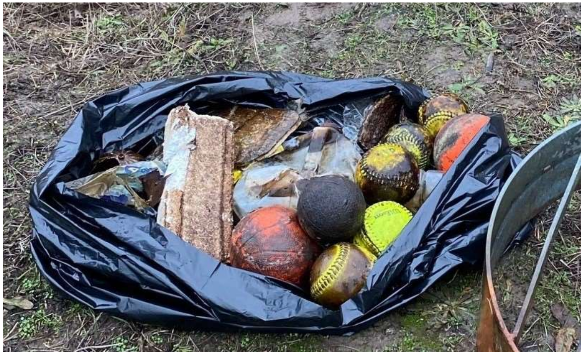
Debris Removed from Outlet
