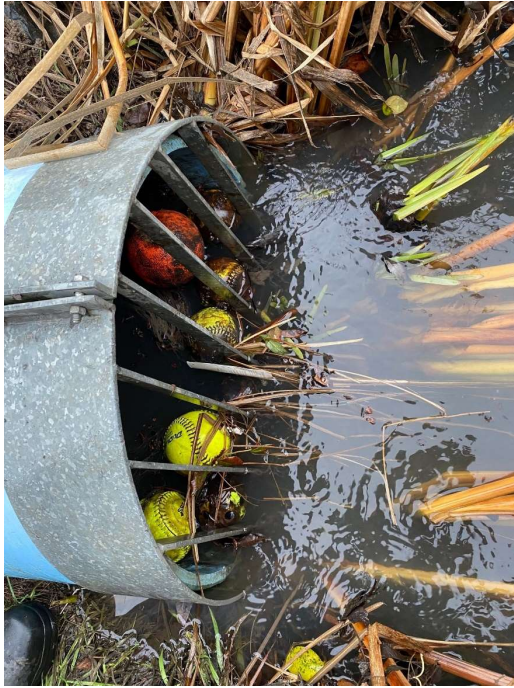
Debris In Outlet Pipe after Leaves Removed
