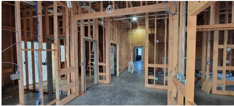
Figure 1: Looking north from the Lobby into the hallway between the Lt. Office and Kitchen
