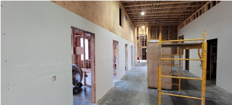
Figure 8: Looking east from the area between the Dorms and Restrooms towards the Meeting Room
