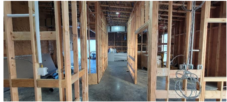
Figure 2: Looking east from the Lobby into the hallway between the Office and Kitchen
